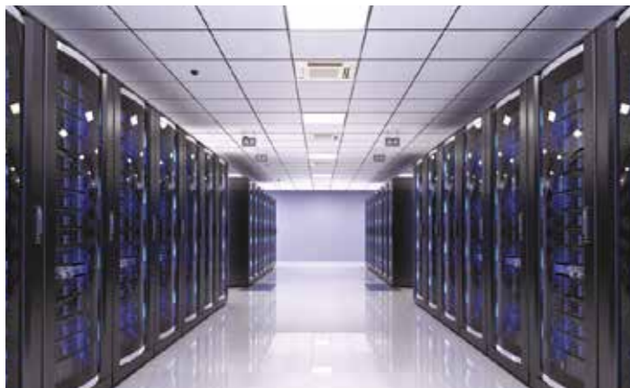
IT & SERVER ROOMS
